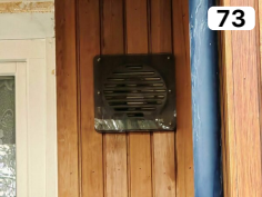
Ventilation (1S69KN) Inspection Type: Intrusive
